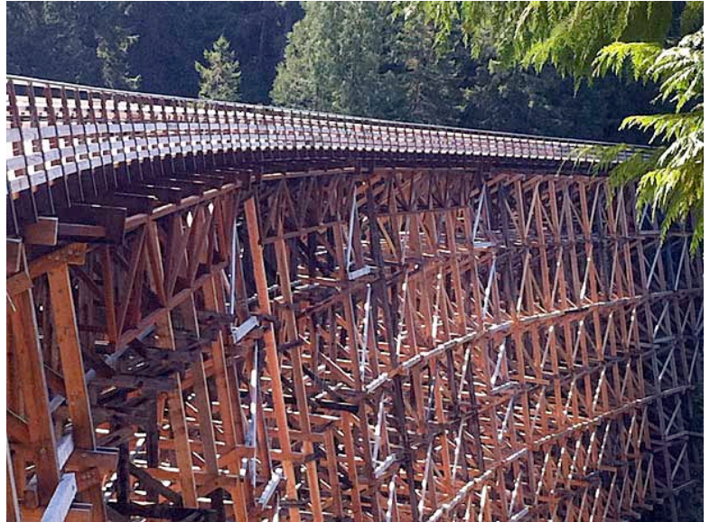
The Kinsol Trestle is one of the largest timber bridges in the world and the highest timber trestle remaining in the Commonwealth at 44 metres high and 188 metres long. (Lisa Cordasco/CBC)
